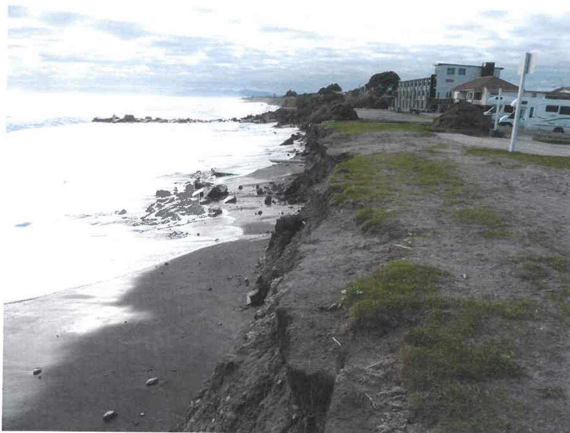
Hokitika Foreshore – King Tide, midday 23 June 2013 Looking North towards Beachfront Hotel. Weld Lane steps in foreground.
