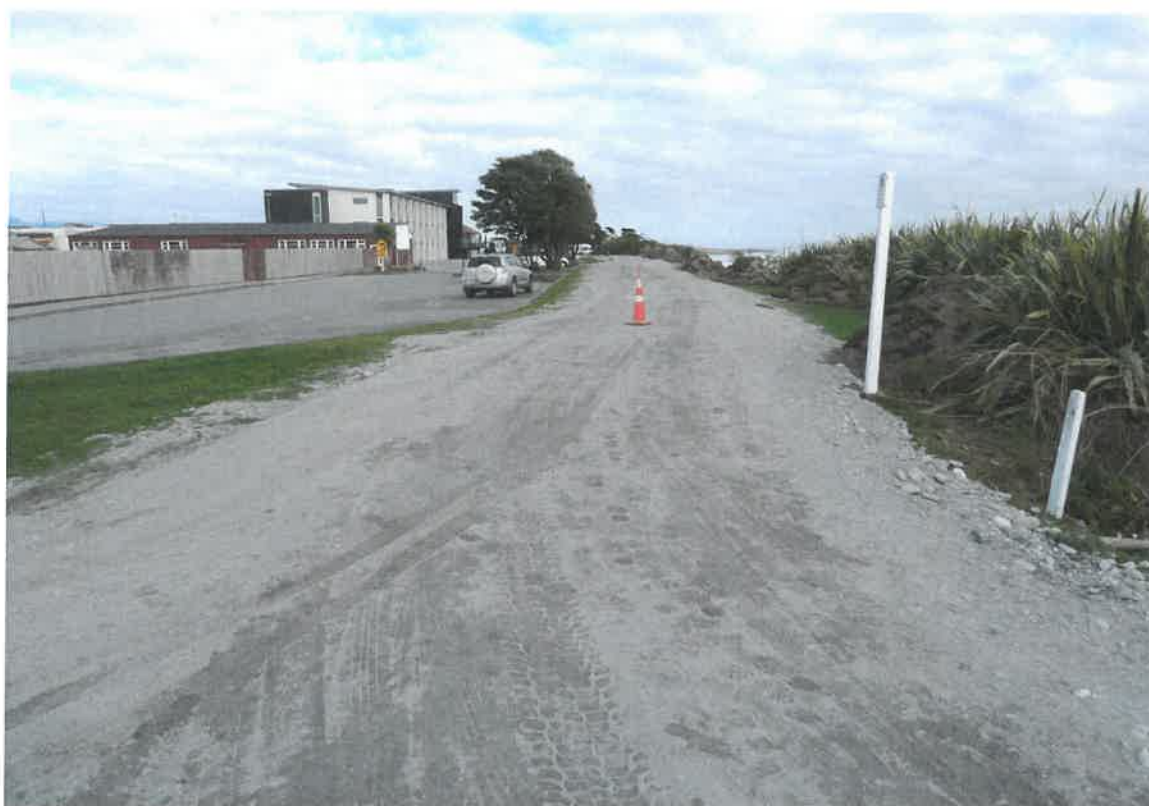
Hokitika Foreshore – Emergency Access Roading - 25 June 2013 Looking South from Stafford street corner towards Beachfront Hotel
